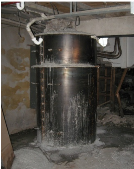
Damaged columns with completed encasement
